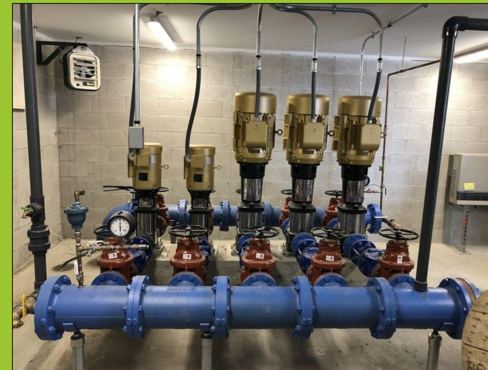
Typical Pumps in a BPS Facility
